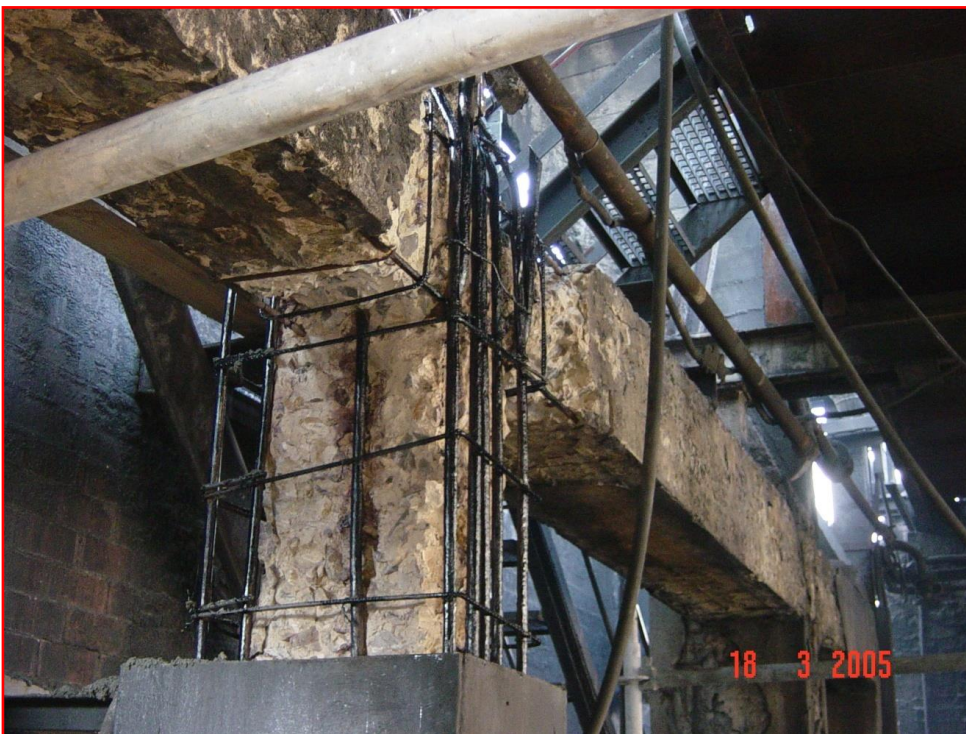
Steel Industry (Coke battery) Asturias SPAIN
